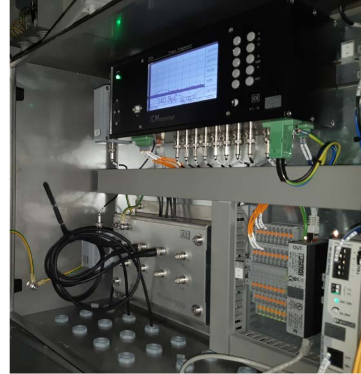
Online PD spot testing/ monitoring with ICMsystem, or ICMmonitor portable, or ICMmonitor
