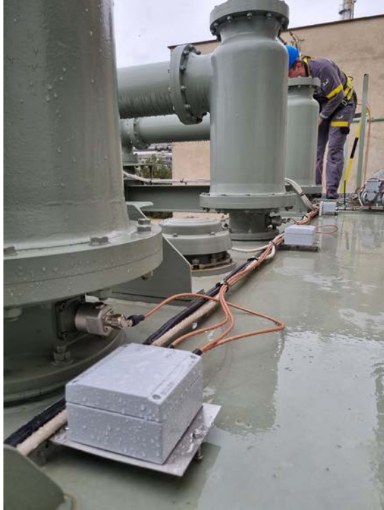
Bushing adapters and bushing coupling units on HV bushings
