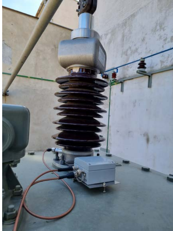
Bushing adapters and bushing coupling unit on HV neutral
