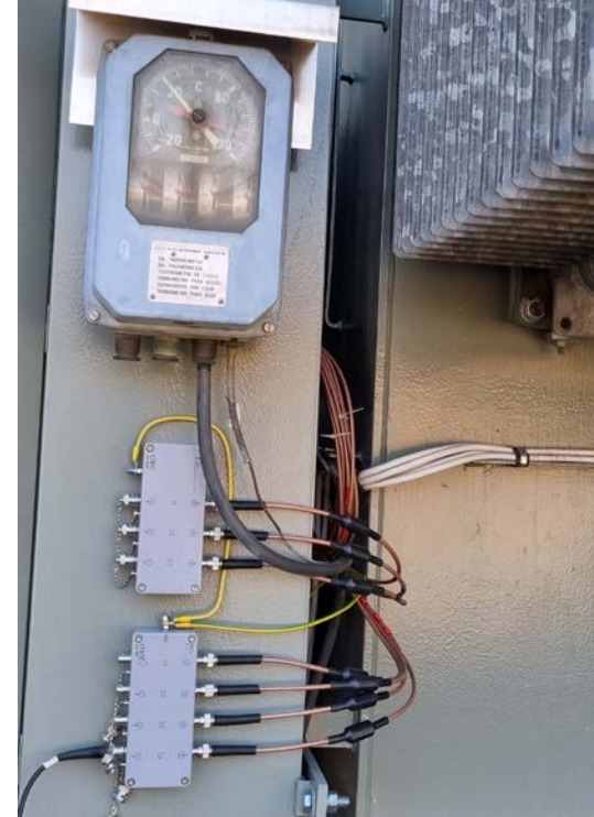
Coupling termination boxes with synchronization and PD signal outputs
