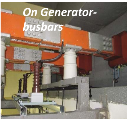
Examples of coupling capacitors installations
