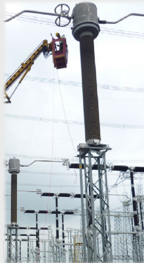
India 765 kV substation
