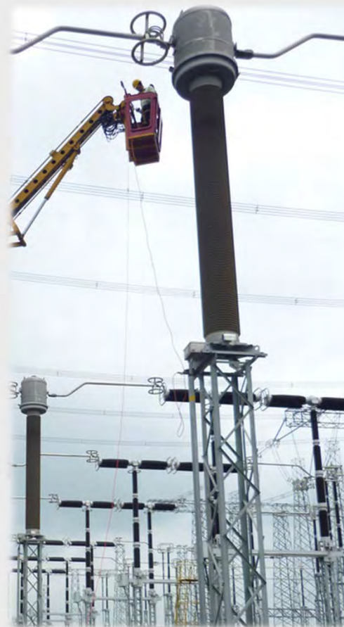
India 765 kV substation
