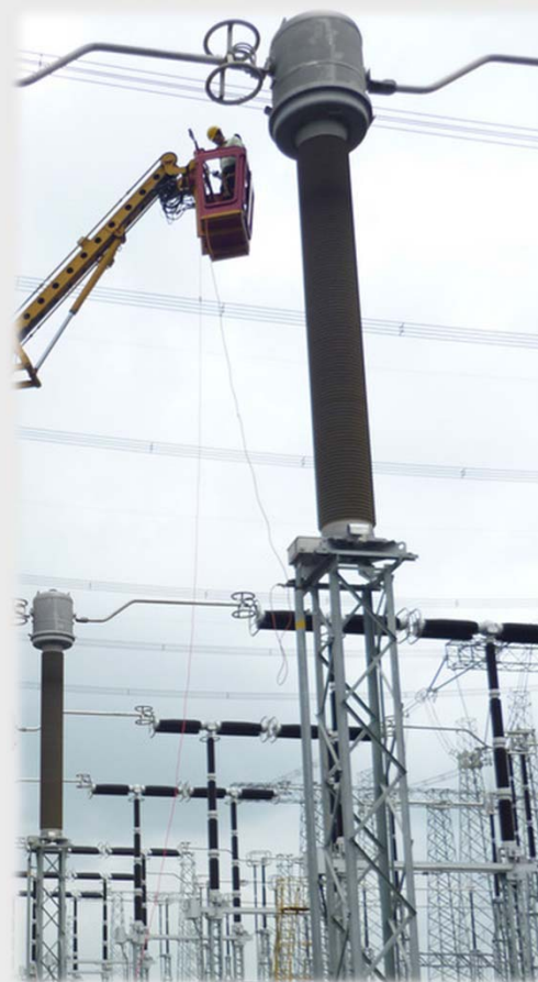
India 765 kV substation
