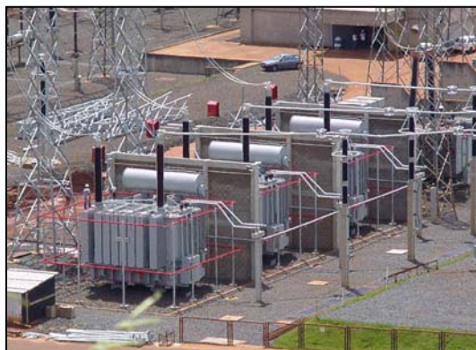
Substation FURNAS, Brazil
