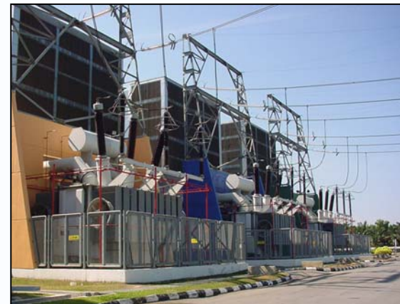
Comb. Gas Power Station Malaysia
